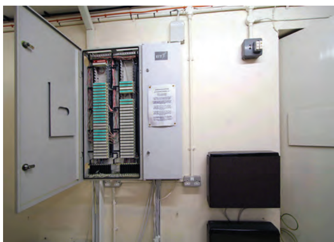
Wall-mounted Line Terminating Unit in the BT equipment room
